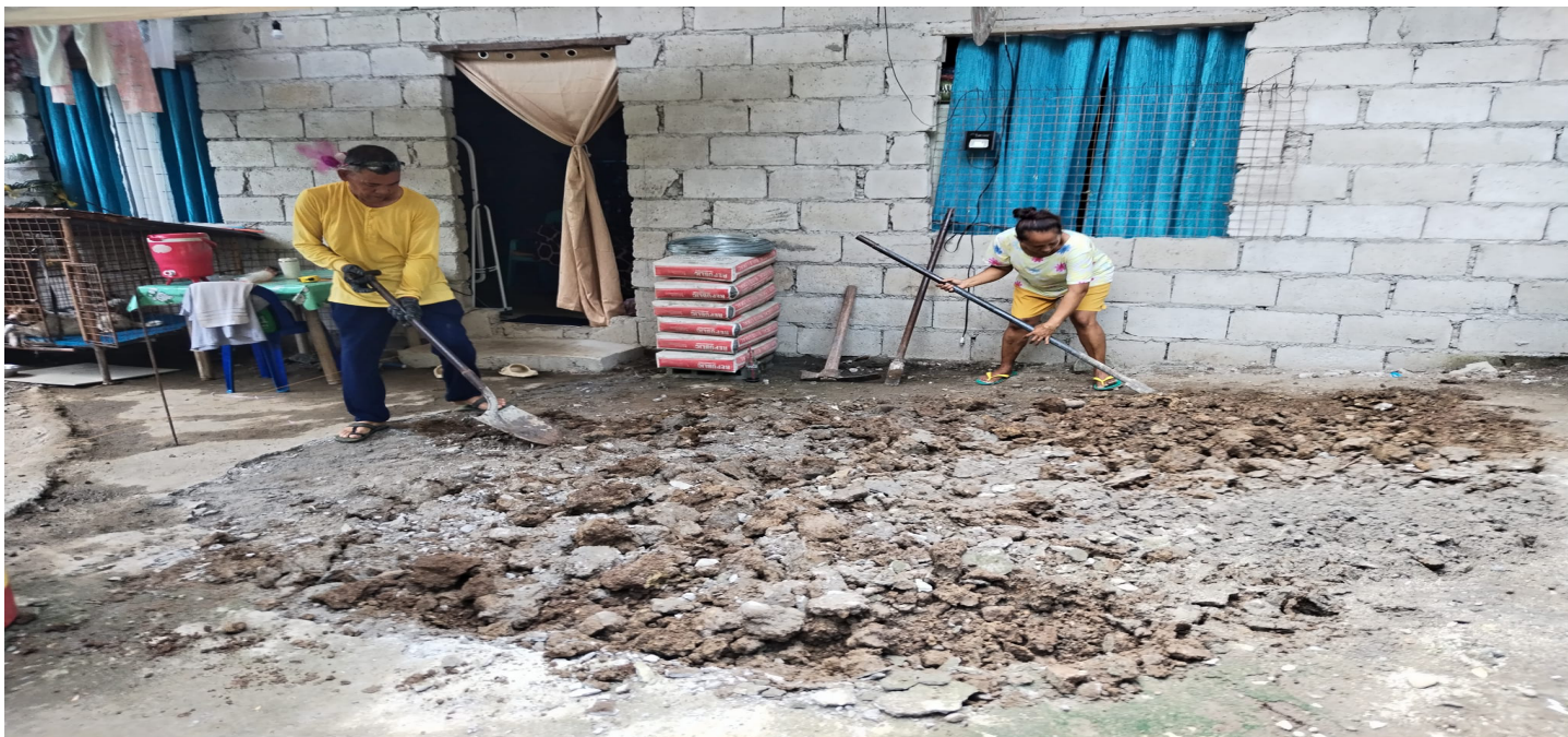
The church family of Pastor Jerome De Castro is helping prepare the front yard to have concrete poured for a temporary place to meet for church.
