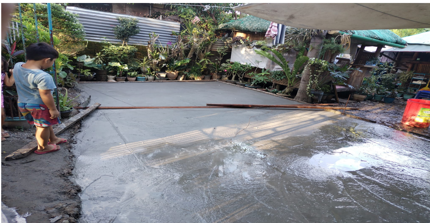
The floor was approaching completion for Pastor Jerome and the church family in the Manggahan area.
